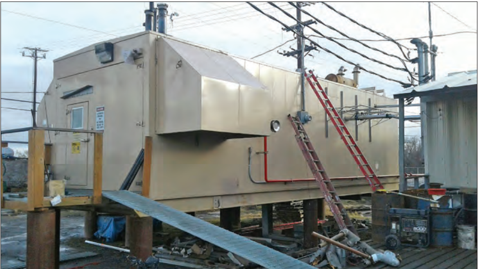
Alakanuk's new standby module.
