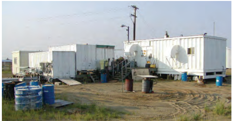
Huslia's power plant.
