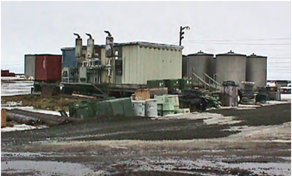
Eek's power plant.
