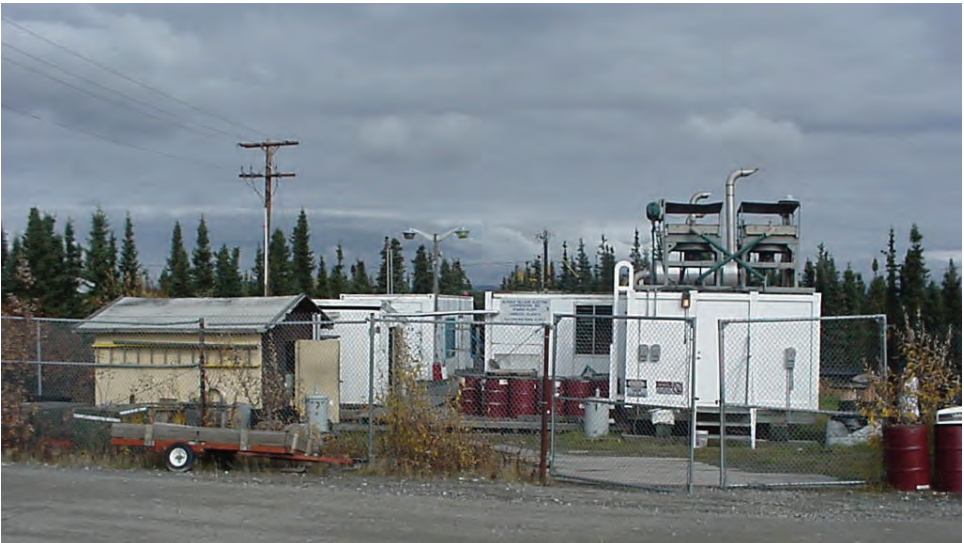
The Ambler power plant.
