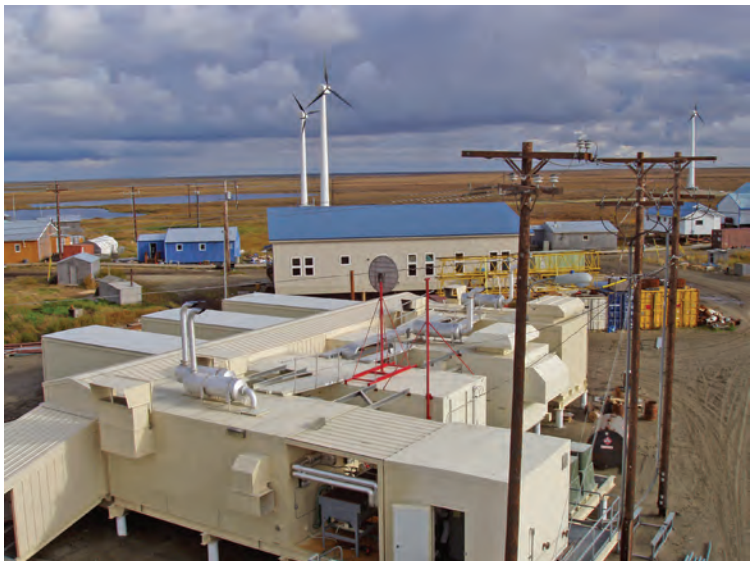
An aerial view of the power plant and wind generators in Kasigluk.
