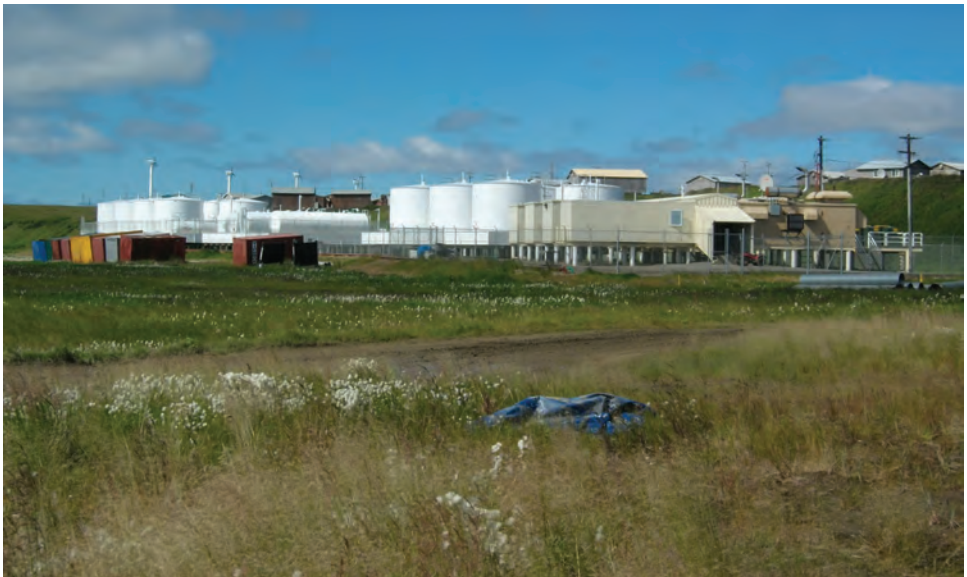
Chevak's new power plant, bulk fuel tank farm and wind turbines.
