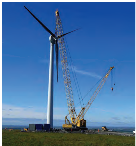
St. Mary's EWT 900 wind turbine.
