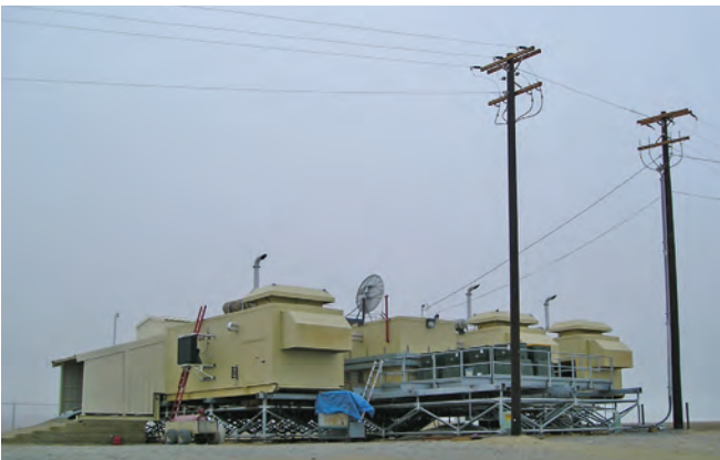
Brevik Mission's new power plant.
