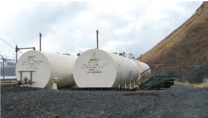
The Old Harbor bulk fuel tank farm.
