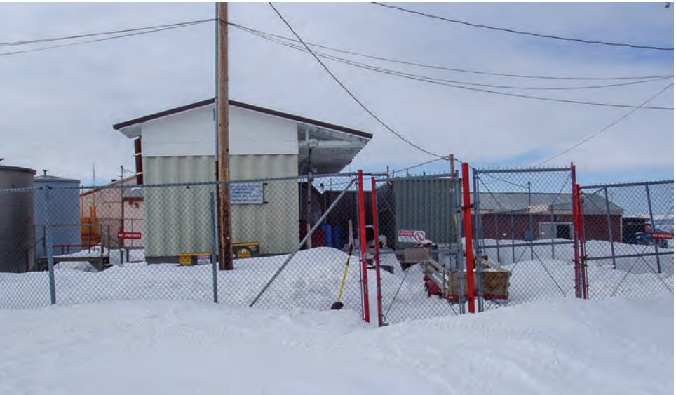
Goodnews Bay's power plant.
