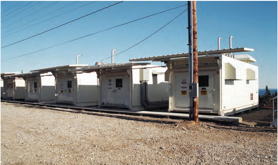
Elim's new power plant.
