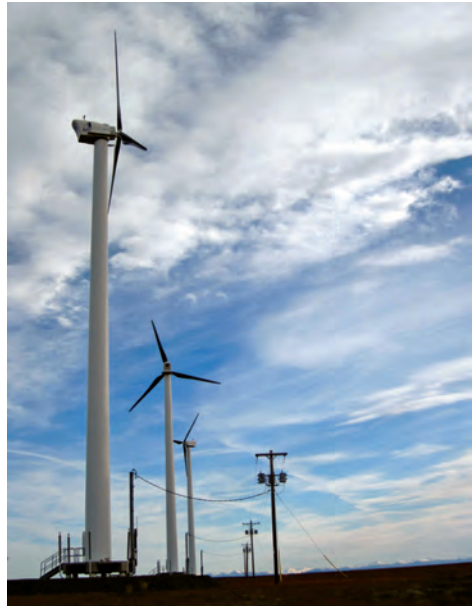
Quinhagak's three wind turbines.
