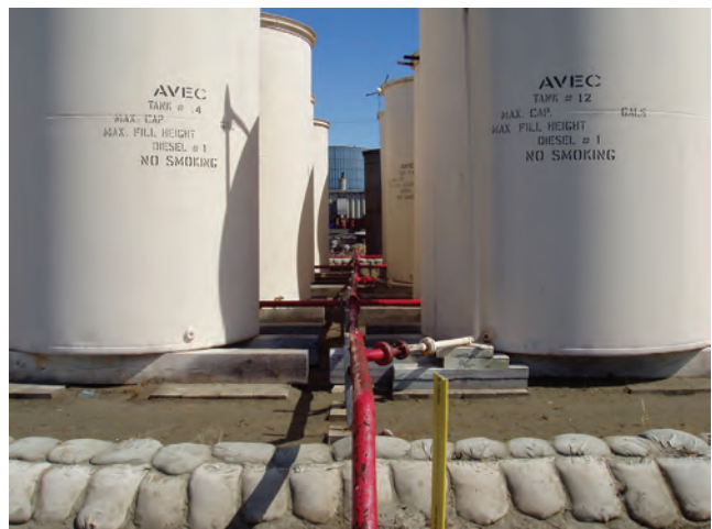
Shishmaref's bulk fuel tank farm.
