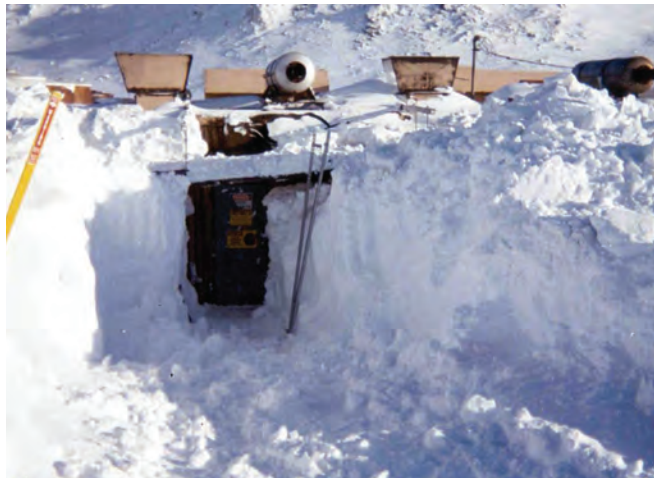
Gambell's power plant buried by snow.
