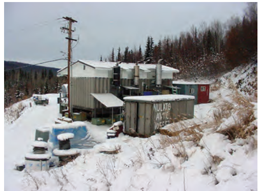
The Nulato power plant.
