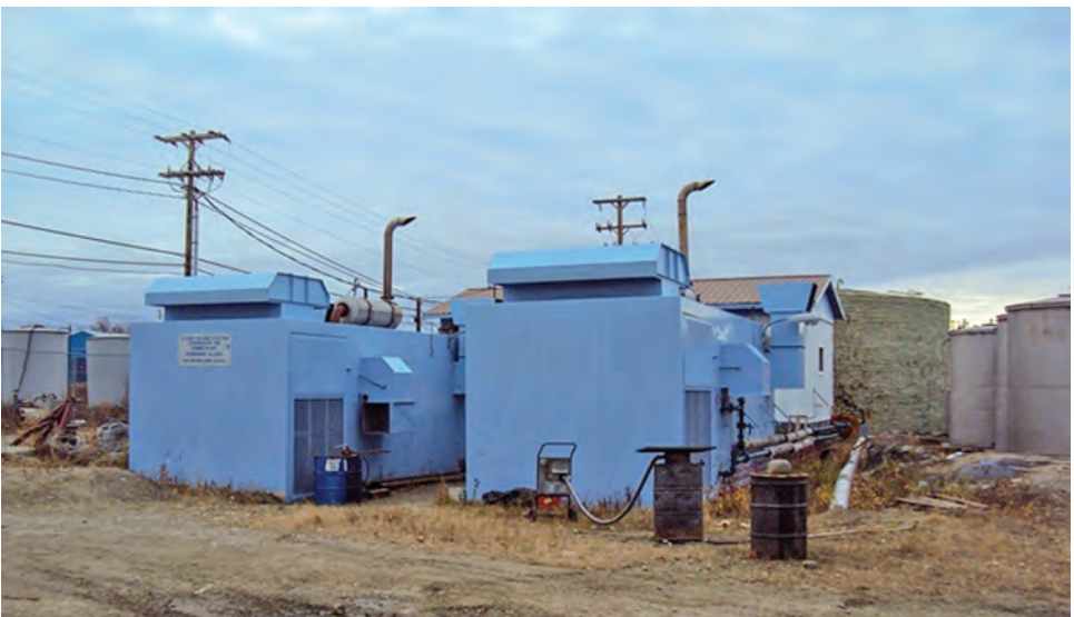
Shungnak's power plant.
