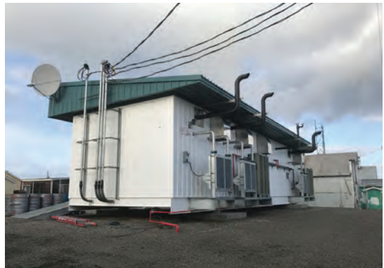
Teller's power plant.
