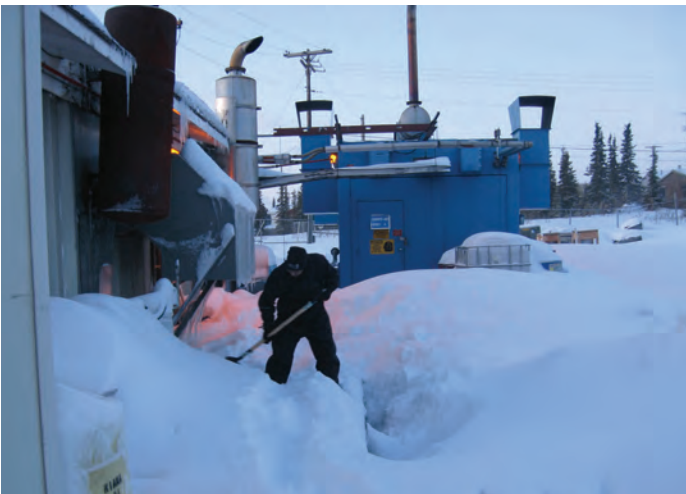
Digging out the Kiana power plant from a deep snow.
