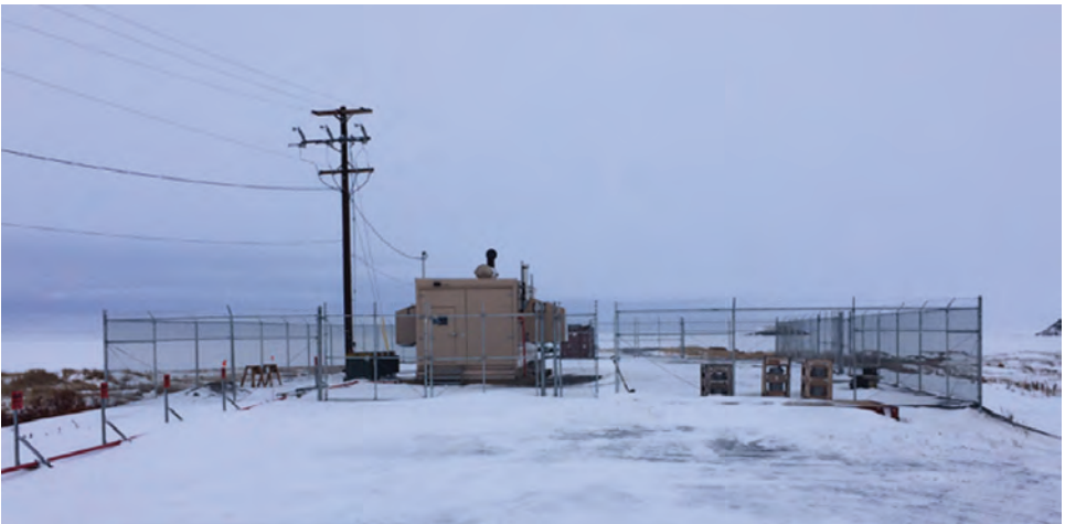
St. Michael's standby generating module.
