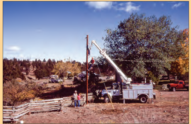
The Nelson Ranch southeast of Prineville was one of the last working ranches in the area to receive power. They were finally connected in the 1990s.
