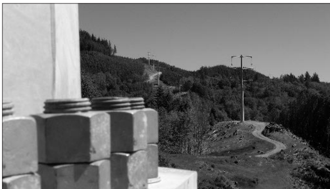
Crews tighten large bolts after steel towers in the Carpenterville Road area are set in place in June 2010 during the final phase of the transmission line upgrade project.
