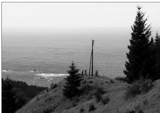
Gold Beach line crew installs a new pole in an area off Carpenterville Road accessible only on foot.
