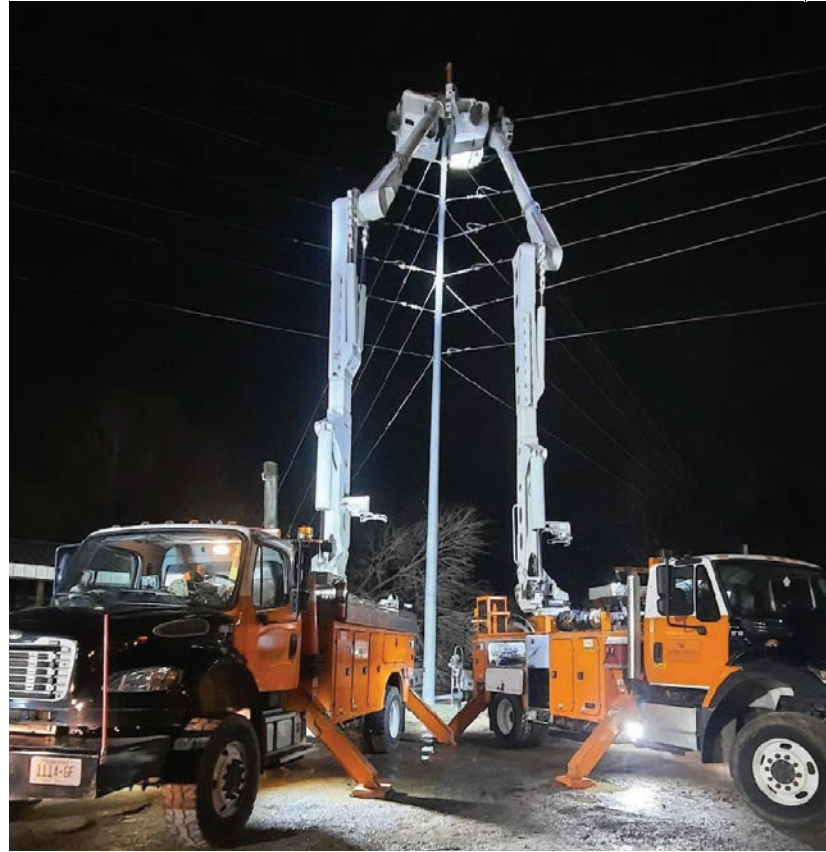
Sevier County Electric System assists with restoration following a 2021 tornado in Mayfield, Kentucky. PHOTO COURTESY OF SCES
