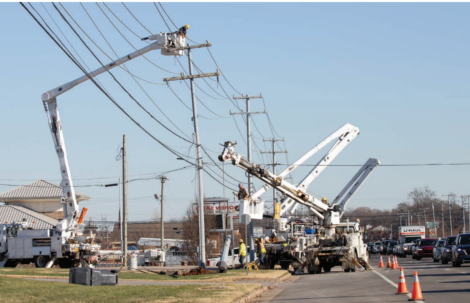
When a tornado struck Clarksville last year, 40 additional line crews—more than 300 workers—joined the tireless effort to rebuild the electric infrastructure and restore power. PHOTO COURTESY OF CDE LIGHTBAND
