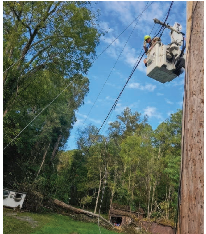
Tullahoma Utilities Authority lineworkers help restore power in Elizabethton after Hurricane Helene. PHOTO COURTESY OF TUA
