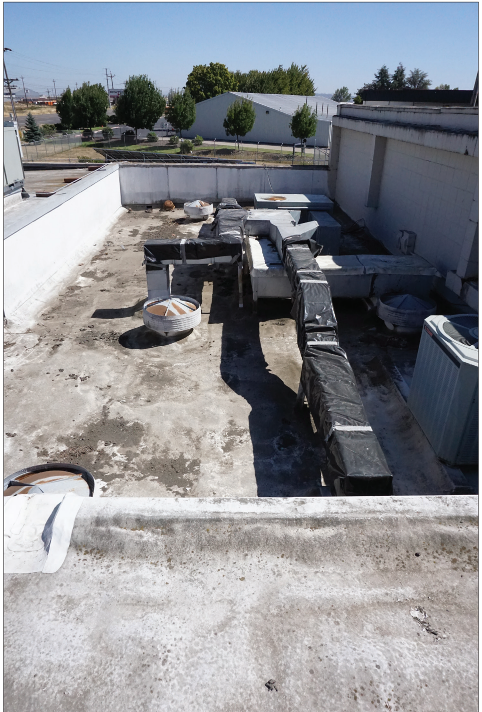
Current three-layer roof does not meet code requirements and is tarped to reduce internal leaks.
