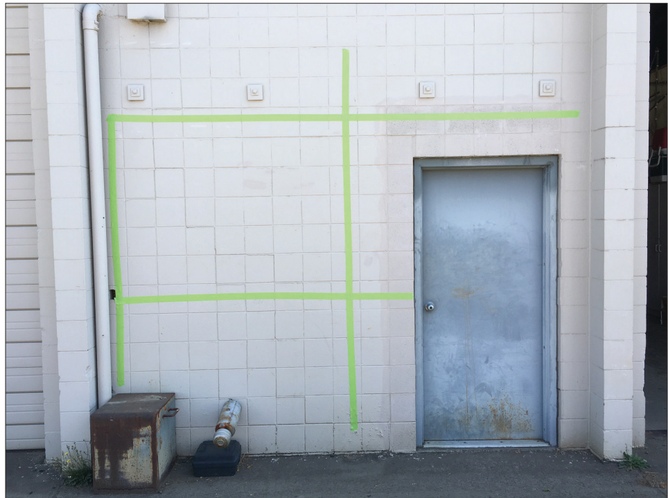
Rebar supports are inadequate for seismic stability of block building.
