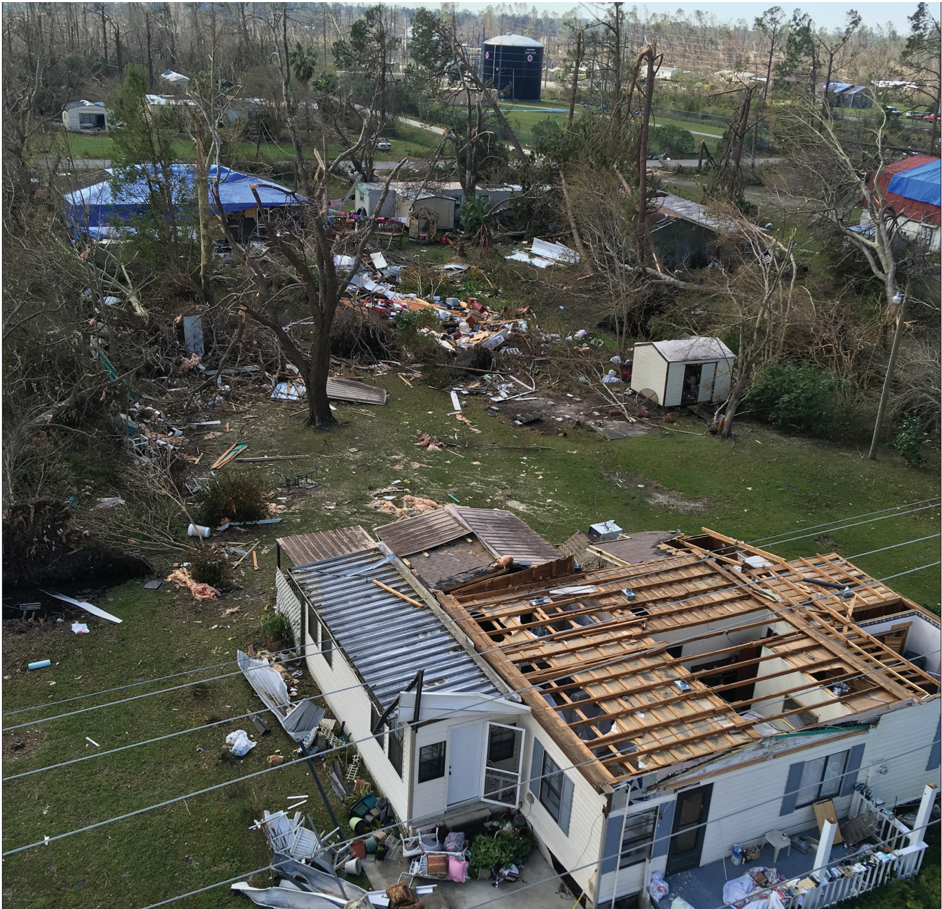
This Panama City home near County Road 2321 was one of thousands destroyed by Hurricane Michael. Blue tarps in the background cover other roofs.
