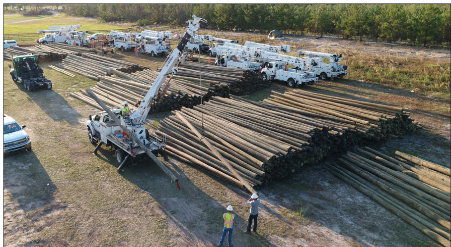
Bucket trucks line up to load some of the 10,000 poles needed to rebuild Gulf Coast's distribution system.
